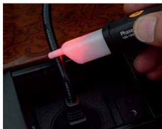
Incorrect phase sequence
